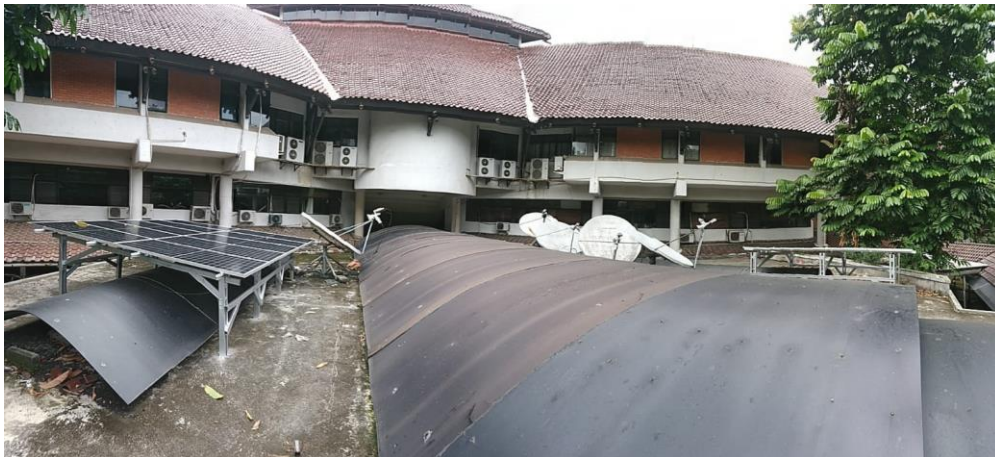
Gambar 3.5. 13 Solar Panel di atap Taman Bougenville
