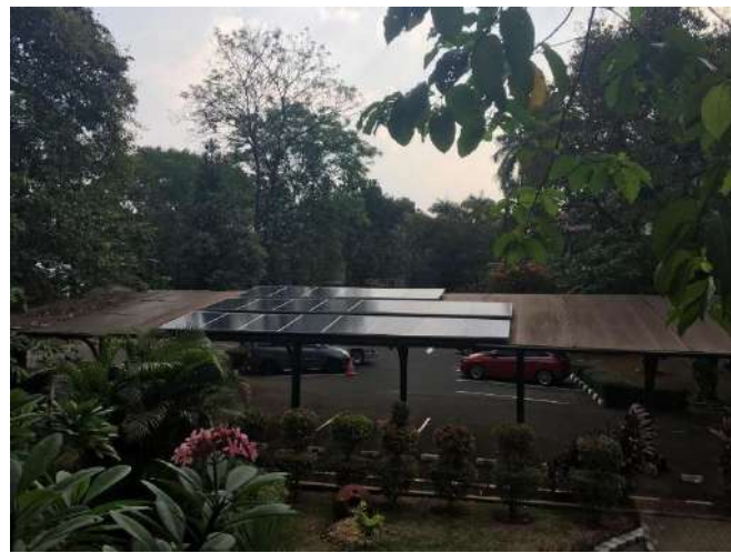
Gambar 3 Solar Panel FKM UI di atap parker mobil Pimpinan
