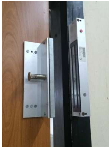
Automatic Door Lock System di Ruang Kerja
