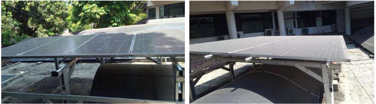
Solar Panel di Lobby A/Taman Bougenville FKM UI
